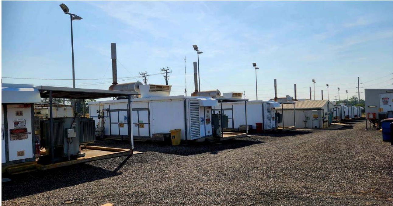
Image 1: Moranbah Power Station.
